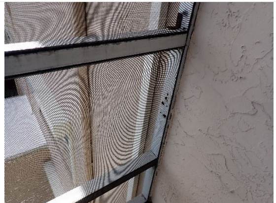
Photograph 8: B345 UNSAFE ~20" opening
