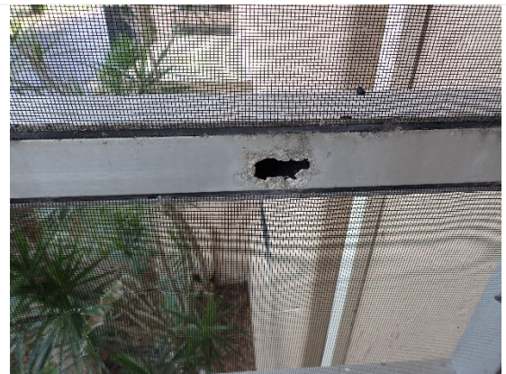
Photograph 6: Pitted Aluminum Guard
